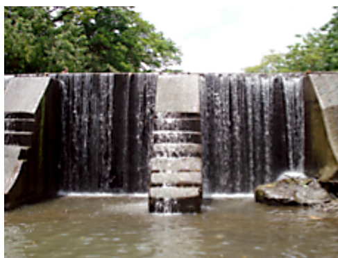
FIG. 3. Weir separating Masachapa river from estuary.
